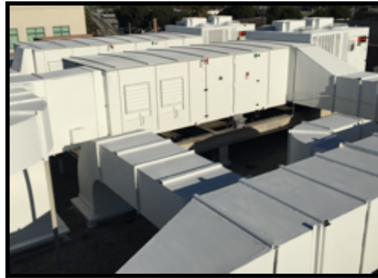
Thermal Barrier for HVAC & Duct Work
