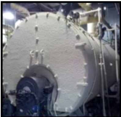
Boiler and Pipe Insulation
